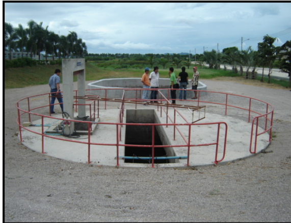
Figure 3 Wastewater collecting tank.
