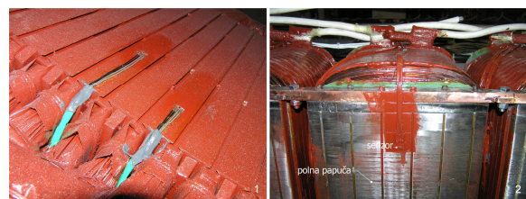
Fig. 5. a) Probes for measuring of magnetic induction in the air gap installed at the stator core tooth,
