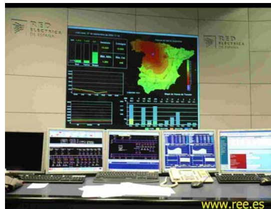
Fig. 5. General view of the CECRE.
