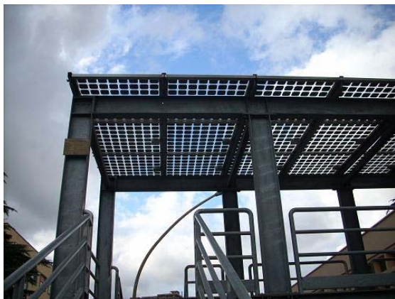
Fig. 1. View of the PV array
