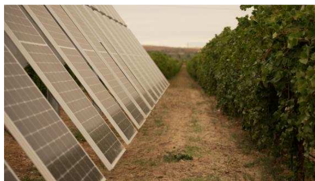
Fig. 4. Installation of smart photovoltaic panels in a vineyard. An example of how renewable energy generation coexists with the rural environment.
