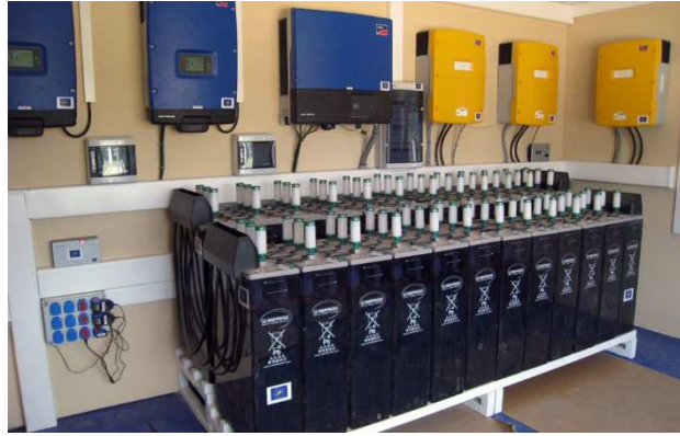
Fig. 1. Batteries and inverters associated with a stand-alone solar photovoltaic system. Barbastro (Zaragoza, Spain).
