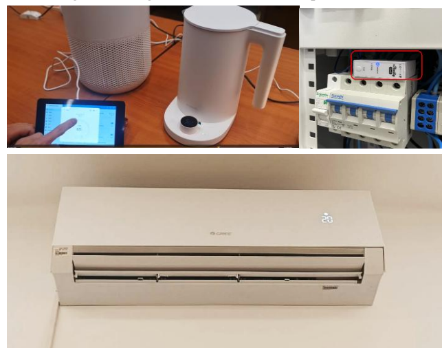
Fig. 4. Water boiler, 3 phase meter for PV metering and air conditioner
